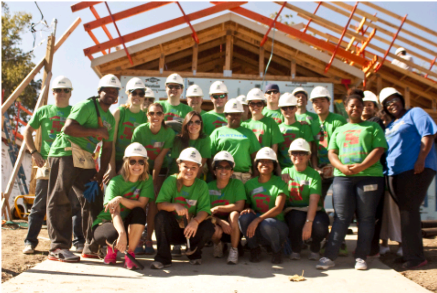
Westwood's Annual Habitat for Humanity Build; Employees volunteer every year to build a home for Habitat for Humanity, just one of the many organizations we serve. (Photo: Business Wire)
